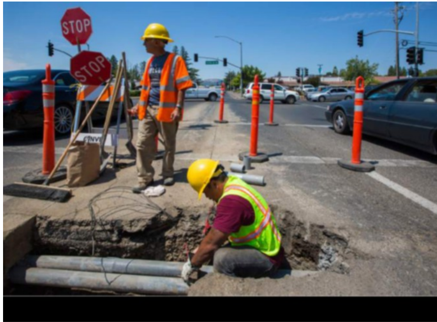
Caltrans workers responded swiftly to the report of traffic lights completely nonfunctioning at the Fifth Street West and West Napa intersection. (Phot by Robbi Pengelly/Index-Tribune)
