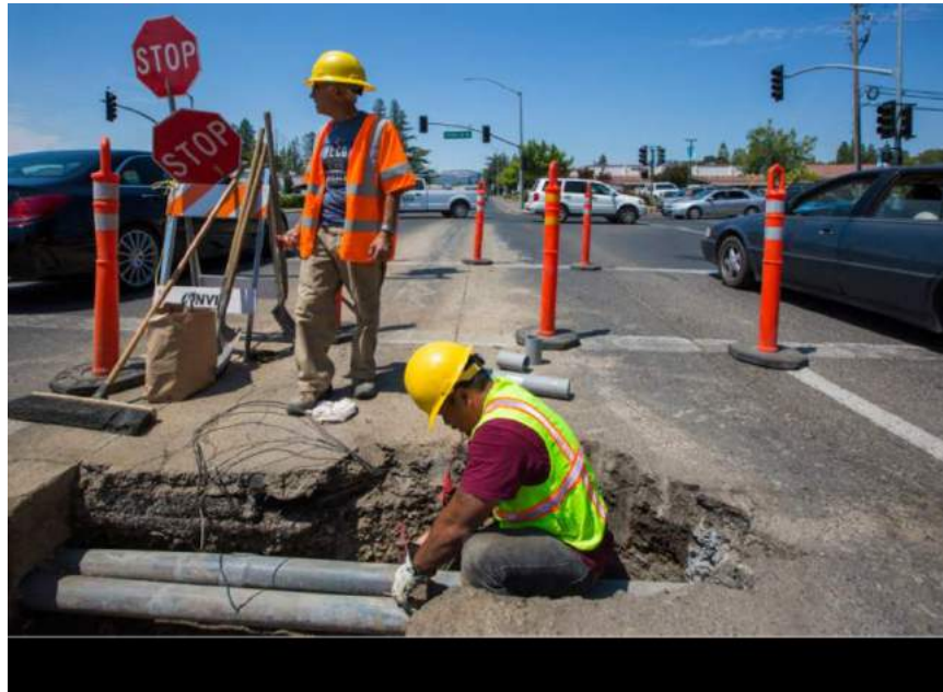
Caltrans workers responded swiftly to the report of traffic lights completely nonfunctioning at the Fifth Street West and West Napa intersection. (Phot by Robbi Pengelly/Index-Tribune)
