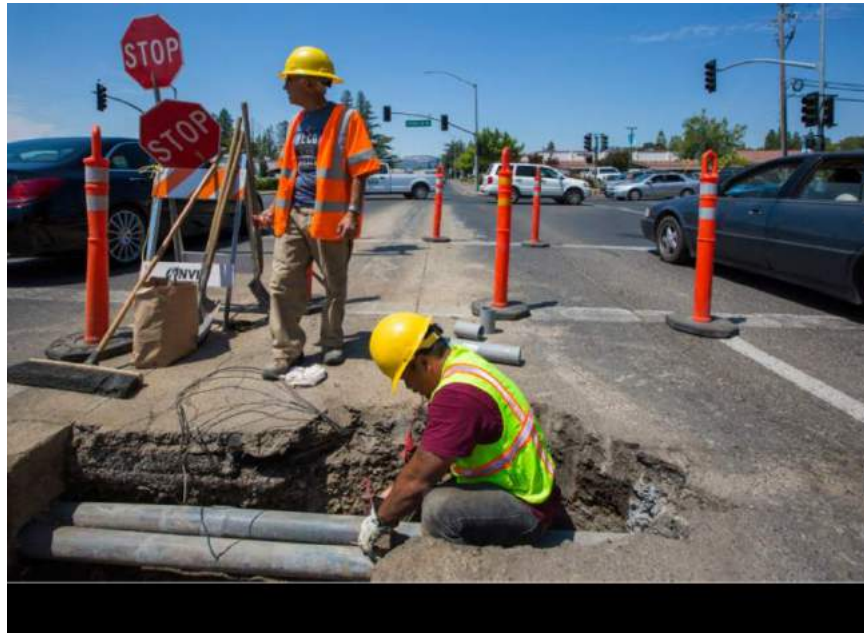
Caltrans workers responded swiftly to the report of traffic lights completely nonfunctioning at the Fifth Street West and West Napa intersection. (Phot by Robbi Pengelly/Index-Tribune)
