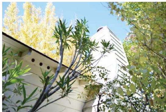
Figure 3: Visible portion of east facade. Rafter tails, vents, and chimney clad with lapped wood siding. Looking northwest.
