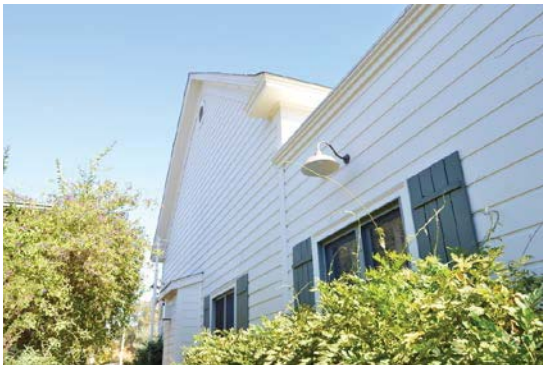
Figure 6: West façade of original portion of barn, with 1998 flat-roof addition to right (south). Looking north.
