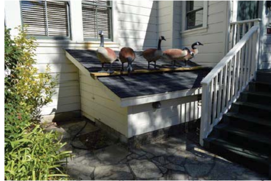
Figure 14: Rear cellar access with shed roof attached to rear facade. Looking northeast.
