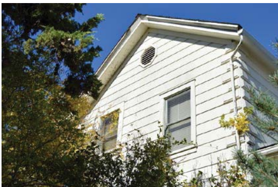
Figure 17: One-over-one double-hung windows at southwest gable end. Former location of brick chimney. Gable vent non-original. Looking northwest.
