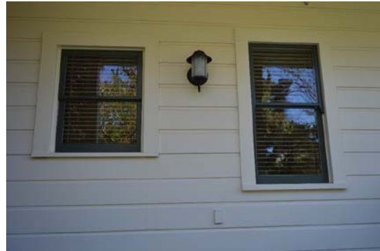
Figure 21: Typical one-over-one, wood-sash windows found at west and south façades (not visible from street) of Burris House. Looking east.
