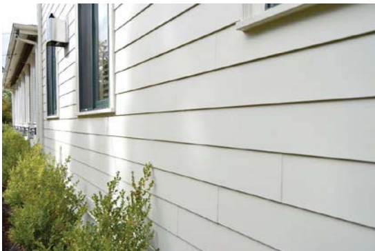
Figure 8: View of Masonite siding along south facade of barn. Typical cladding material found on non-original portions of barn. Looking west.
