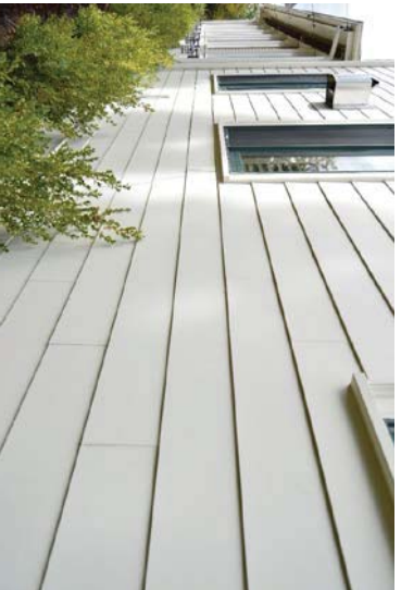
Figure 31: View of Masonite siding along south facade of barn. Typical cladding material found on non-original portions of barn. Looking west.
