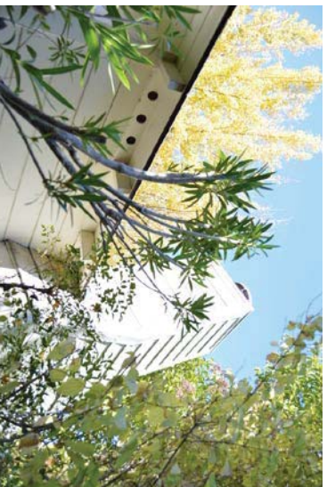
Figure 36: Visible portion of east facade. Rafter tails, vents, and chimney clad with lapped wood siding. Looking northwest.
