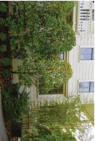
Figure 8: Fenestration at first story of outermost bays at primary (north) façade. Looking south.
