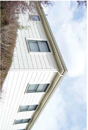
Figure 41: Second story of central, two-story volume of pool house and spa building.
