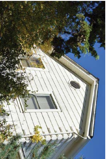
Figure 19: One-over-one double-hung windows at southwest gable end. Former location of brick chimney. Gable vent non-original. Looking northwest.
