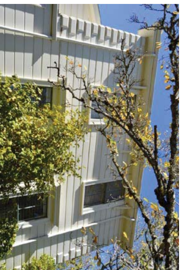
Figure 11: West façade at main residential volume. Rusticated quoins pictured at north and south end of façade. Looking west.
