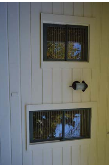
Figure 23: Typical one-over-one, wood-sash windows found at west and south façades (not visible from street) of Burris House. Looking east.
