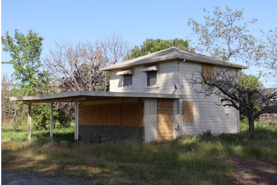
Figure 3. Photo showing the west and south elevations of the ca. 1940 house, facing northeast.
