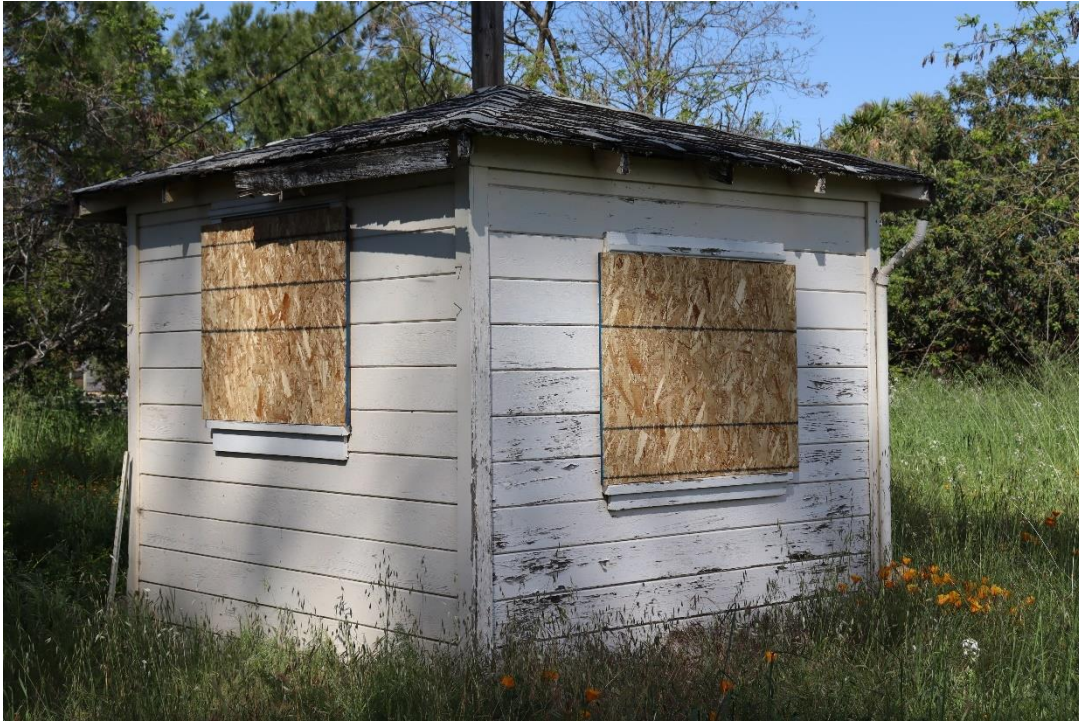
Figure 27. Photo showing the west and south elevations of the ca.1940 auxiliary building, facing east.
