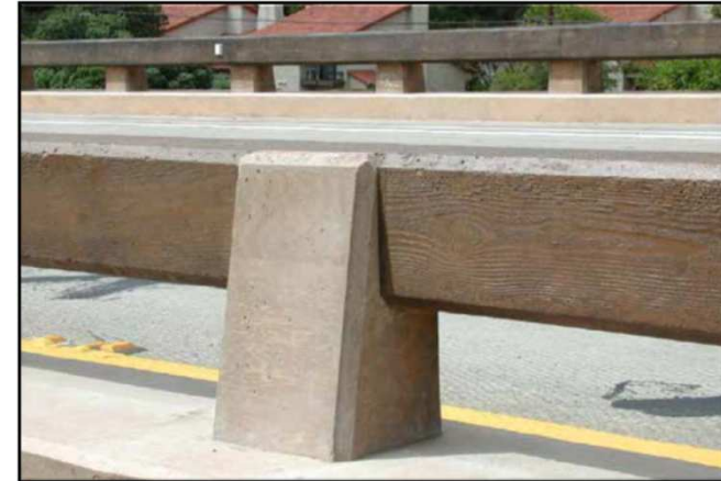
Stained Concrete Bridge Railing
