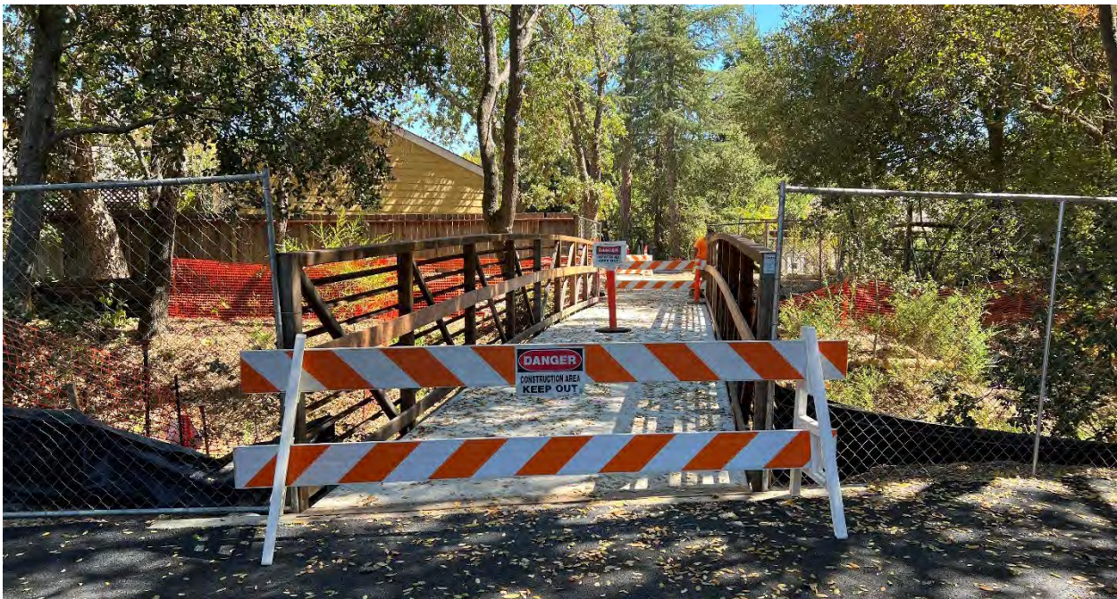
The new Fryer Creek Pedestrian and Bicycle Bridge just before completion, November 2022
