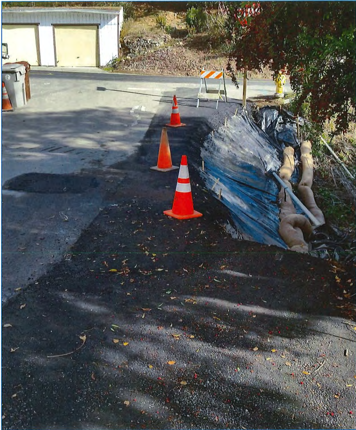
Figure 9: After the sewer pipe was installed in the steel casing and the old pipe was grouted off and sealed, the road was finish paved and then striped. Erosion control in the form of plastic and straw waddles were installed. Work was completed in September 2015.
