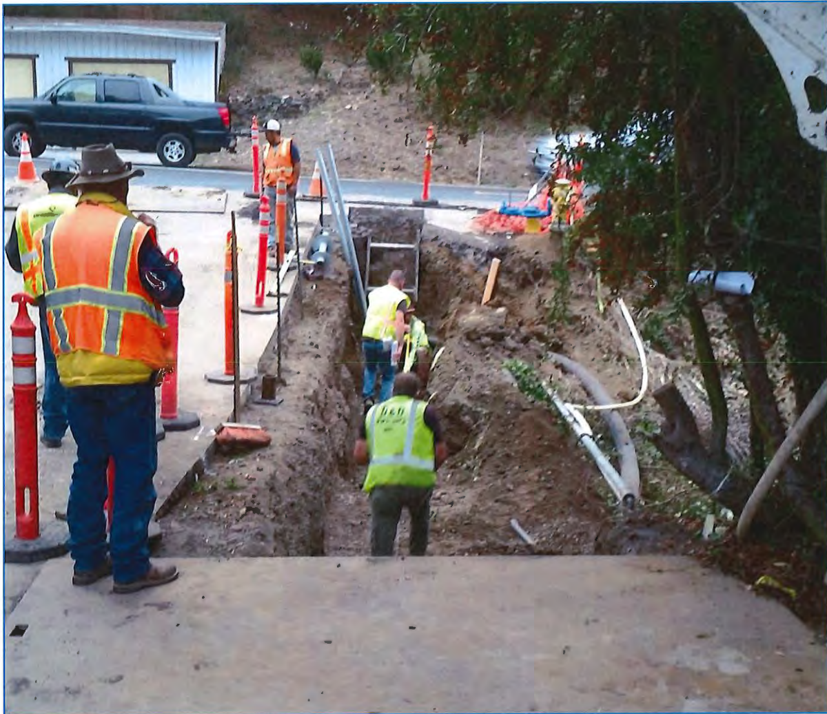
Figure 7: Approximately 1/4 of the AC was removed from Palma way to allow for re-compaction of the sub-base, and the AC was removed an additional 12 to 18 inches to a T-trench per the County of Marin paving standards. This allowed clear access to install the new welded steel casing, August 2015.
