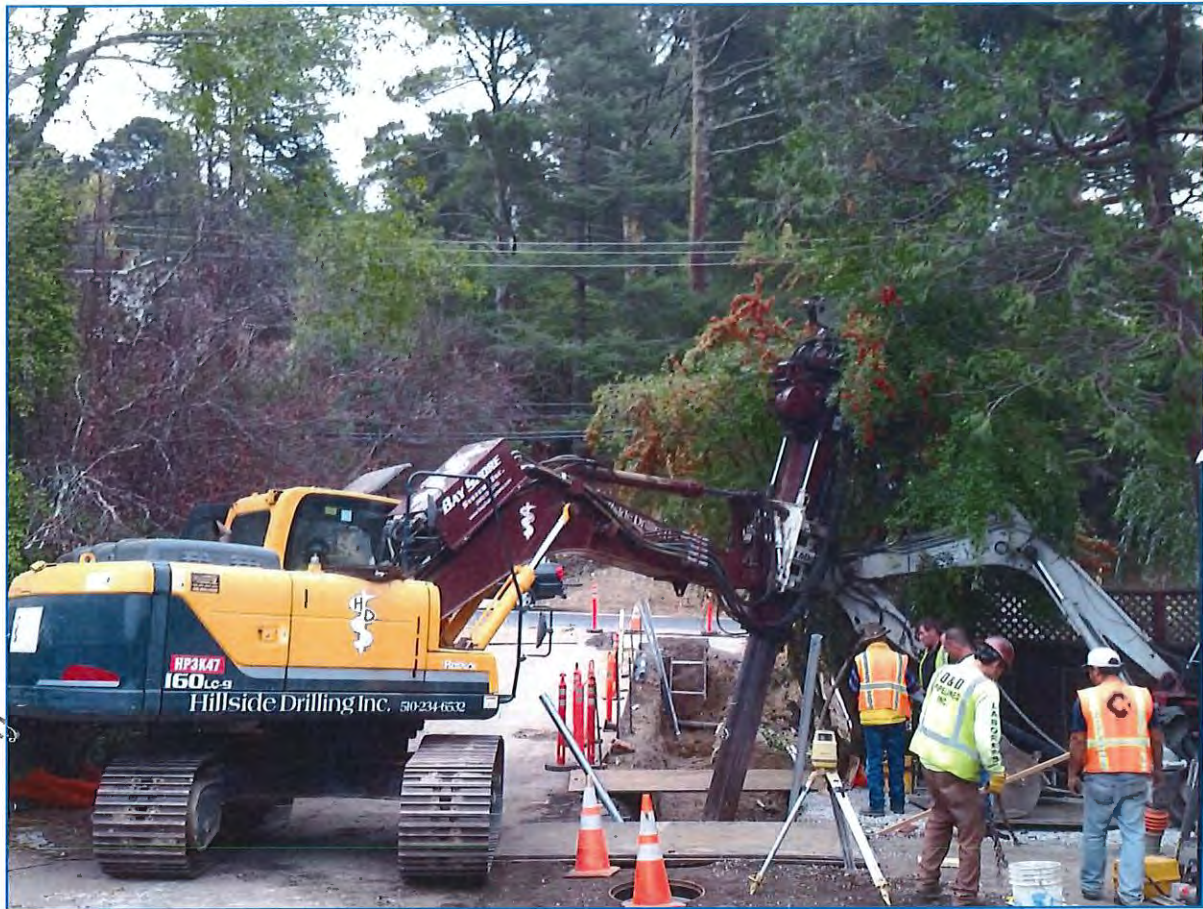
Figure 8: Drilling Machine attached to an excavator, set to drill in the support piers at approximately 15 degrees from vertical. Two end piers angle North, and two center piers angle South, August 2015.
