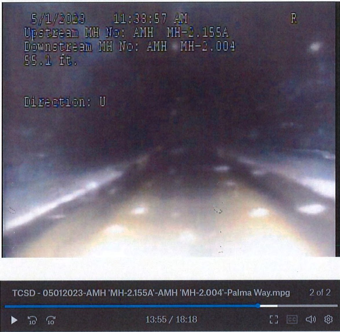
Figure 14: Video capture of the sewer main inside the steel casing mid span over the drainage channel of Palma Way.
