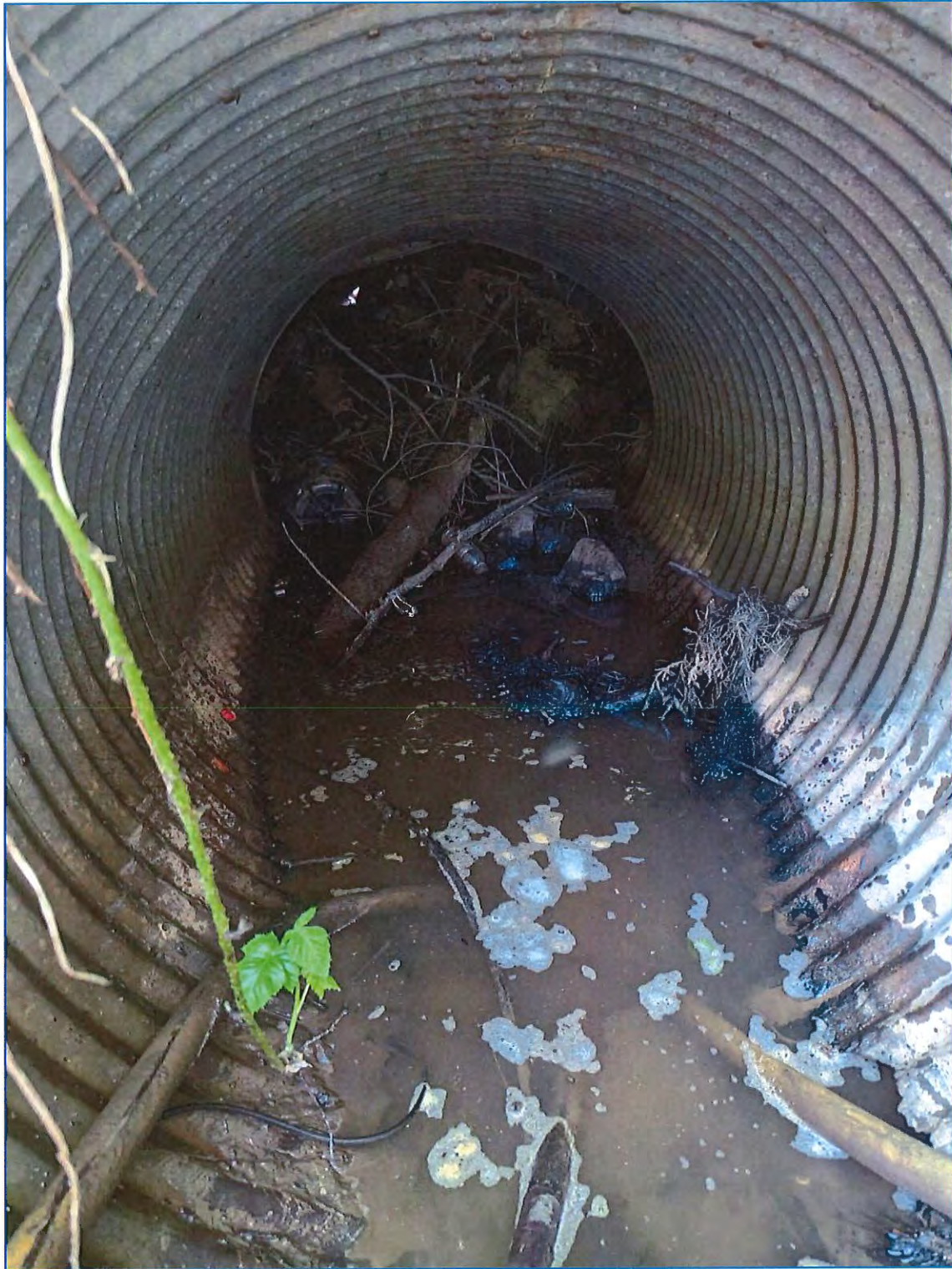
Figure 13: View looking inside the culvert under Palma Way, blocked by debris and rocks. Also the water supply hose was leaking and sitting in septic water which could pose a health risk to residents.
