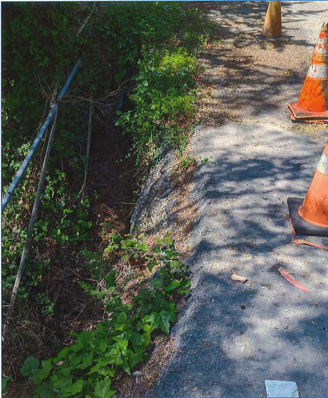
Figure 11: View looking West from Shoreline Highway up Palma Way. The base rock off the edge of the pavement is still in place from the TCSD 2015 sewer repair. Also, the two “fire hose” lines may be water services. There are two water hoses on the South side of Palma Way and two water hoses on the North side.
