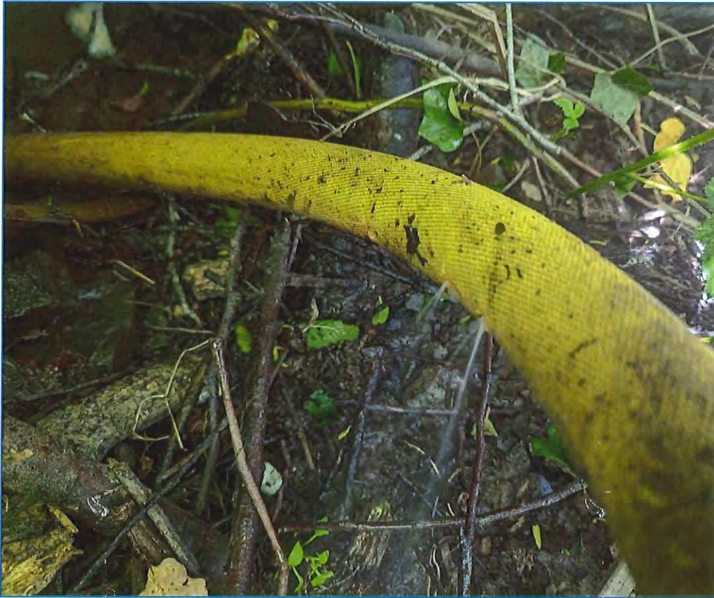
Figure 12: Water leak on one of two hoses serving water to homes on the North side of Palma Way. The forces of the high water and debris may have contributed to hose damage.
