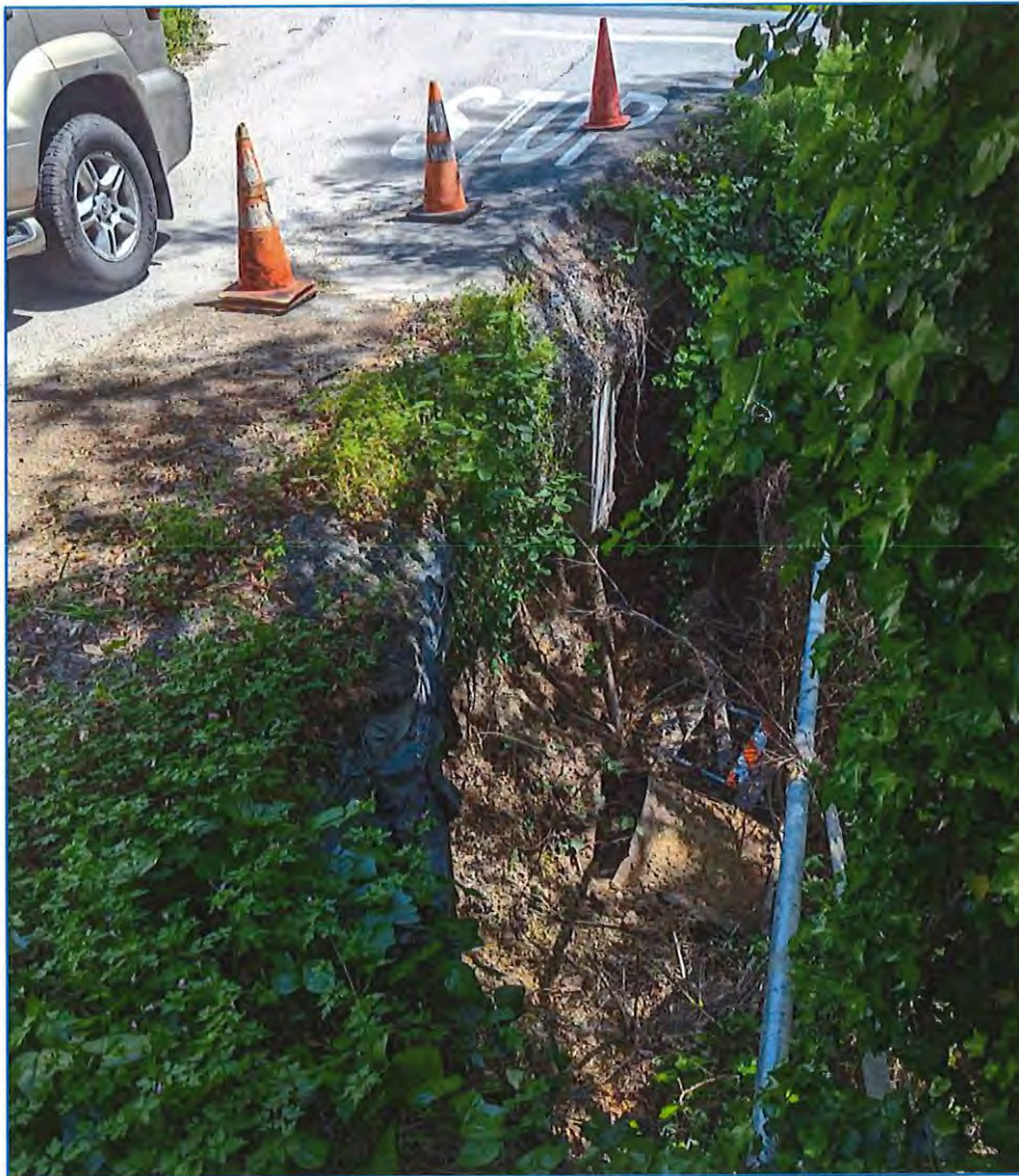
Figure 10: View looking East from Palma Way toward Shoreline Hwy. Compare the location of the silver steel above ground utility that is visible in free span in this image, but was partially buried in Figure 9 above. Also notice the culvert in the middle of the image which has plugged, broken, and tipped down because it was undermined. The concrete block and angled steel pipe visible in the middle of the image is one of the casing pipe supports visible after being exposed.
