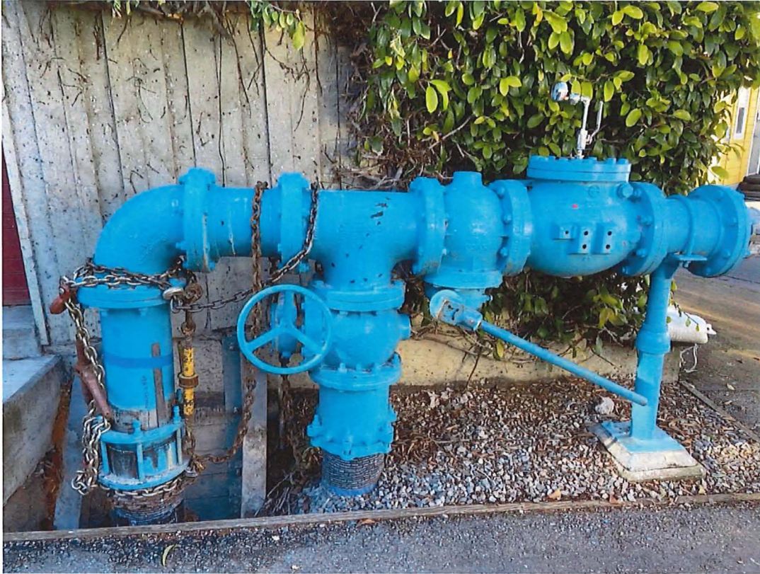
By-pass Valve with chains to stabilize movement
