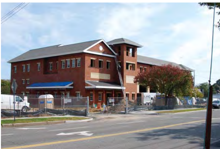
Location 42: View looking southeast toward new institutional fire station along Sunset Ave. in B-1 District
