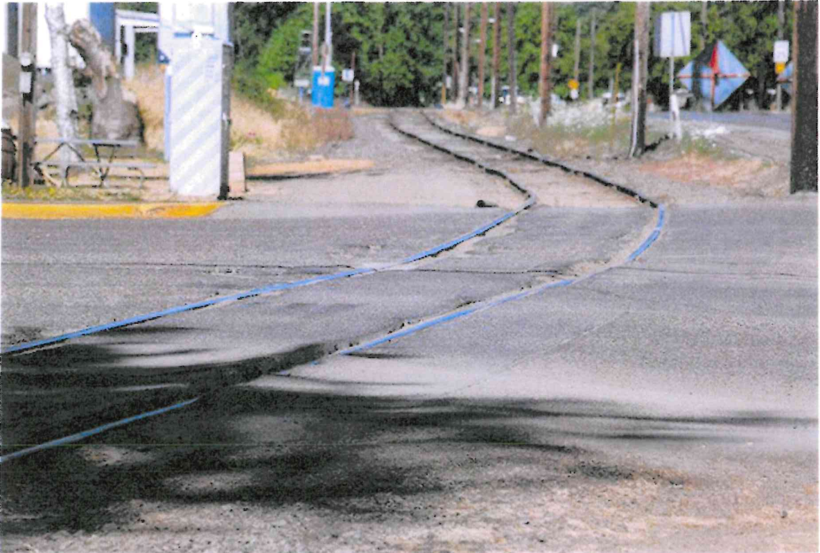
Rusty Rae/News-RegisterWillamina residents believe the railroad crossing on Highway 18 at the west end of town is a hazard, and they want it improved. The Oregon Department of Transportation has proposed a short-term fix.
