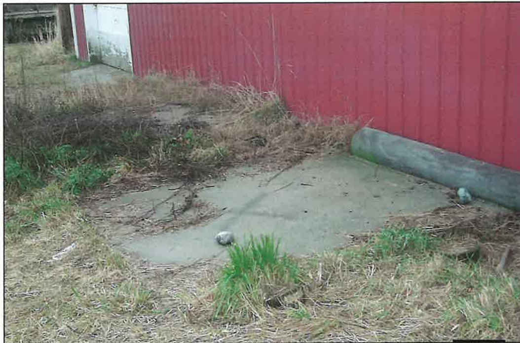
PHOTO NO. 14: Two concrete pads located on the east side of the Elevator building.
