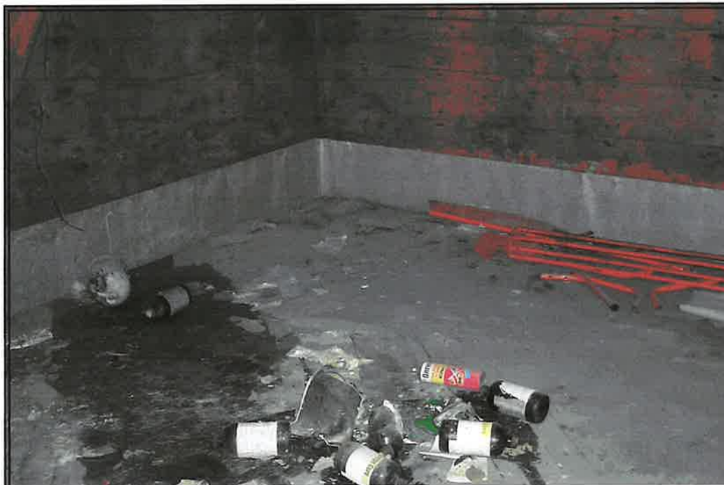
PHOTO NO. 8: Bottles of hog mange located on the second floor of the Elevator building.
