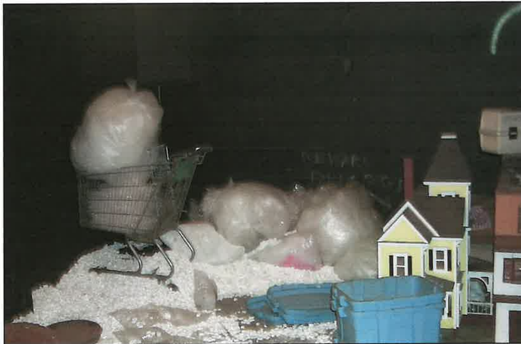
PHOTO NO. 10: Garbage/debris located on the 1 st floor of the Elevator building
