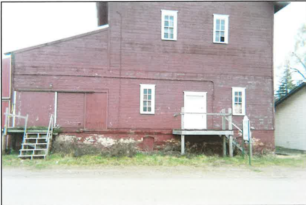
PHOTO NO. 1: The Elevator building located on the north portion of the property.
