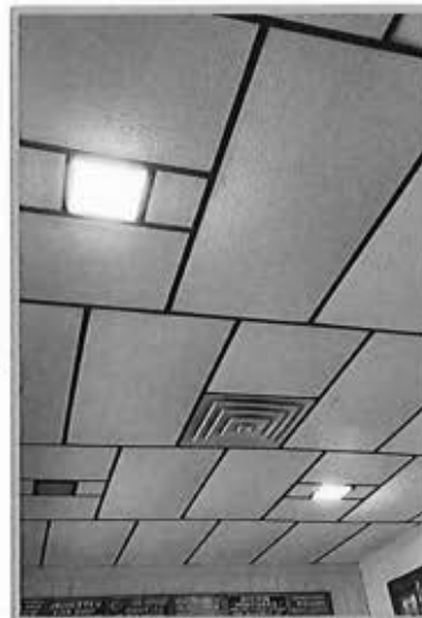
The 1980's drop ceiling in the main room of the Williamston Museum.
