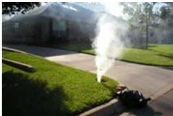
Figure 1. Leaky Pipe Found by Smoke Testing
