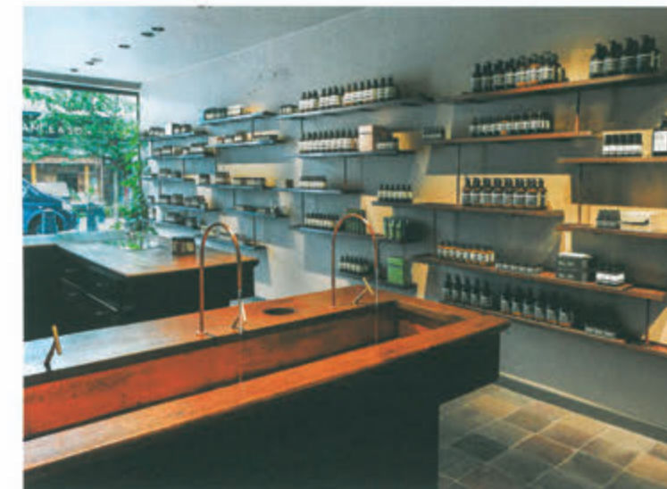
An intricate system of pipes channels water through the shelving at Aēsop in Bloomsbury, London.
