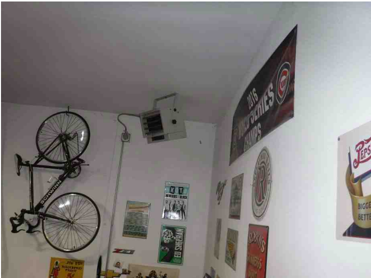
Interior of Garage (Heater)
