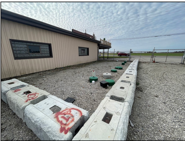
Recently updated septic system
