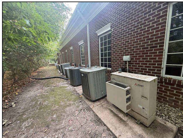
9 ground mounted AC units
