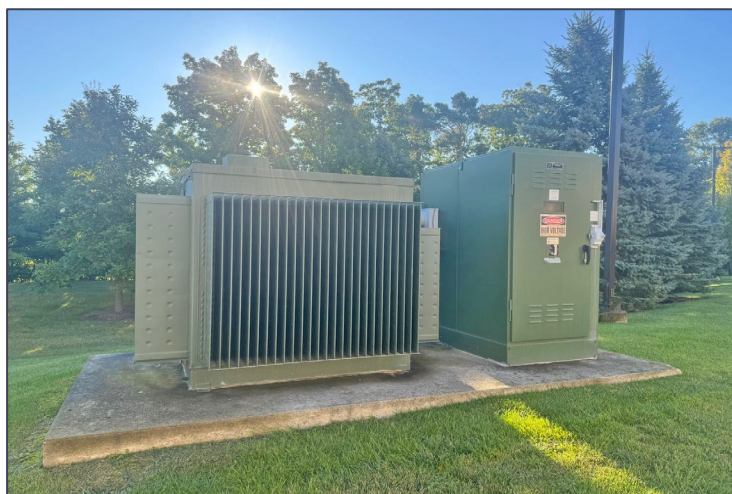
Primary Electric: 2500 KVA Transformer
