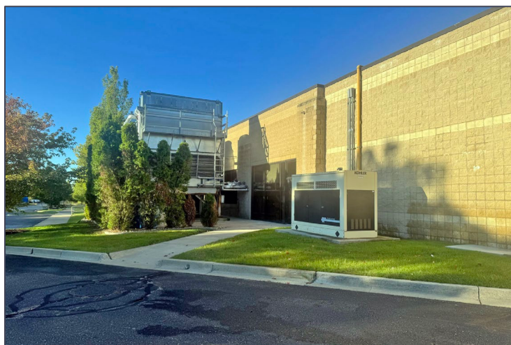
Generator & Cooling Tower
