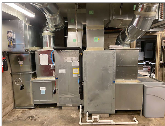
Newer HVAC equipment
