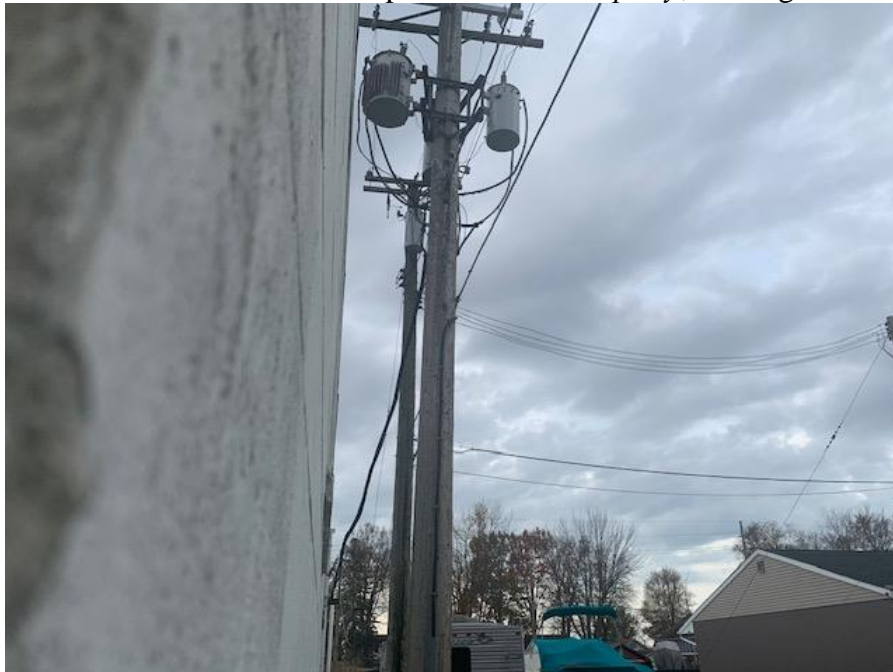
Photo 28. View of pole-mounted transformers just beyond the western Property boundary
