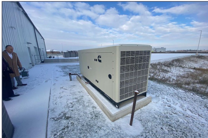
Natural Gas Generator
