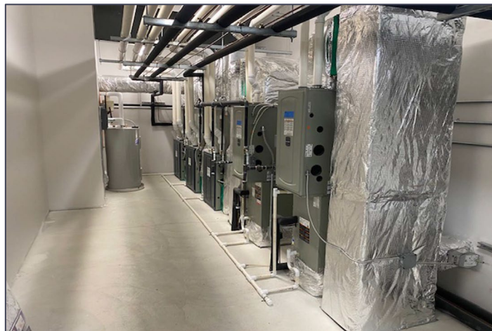
5 HVAC Units Above Office
