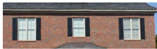
Inappropriately Scaled Shutters: Not Permitted
