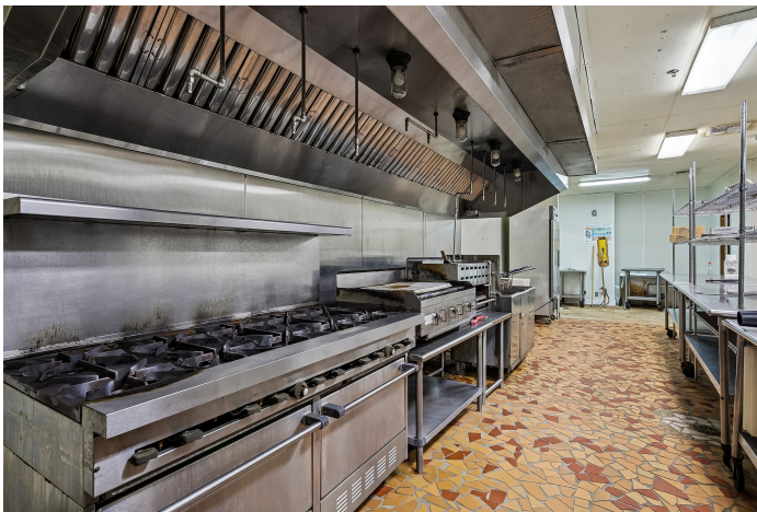
Commercial kitchen and hooded cook line
