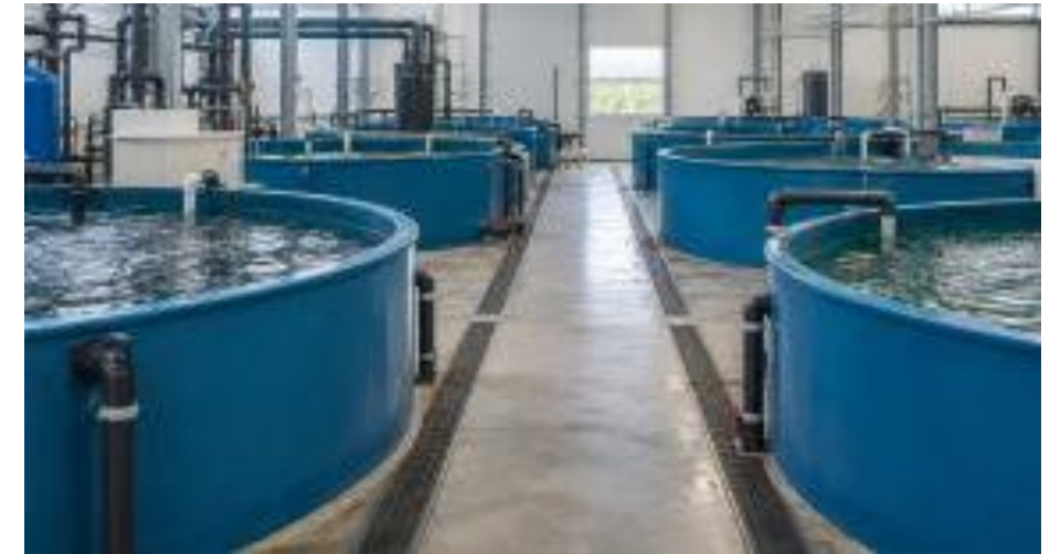
Illustrative RAS facility
