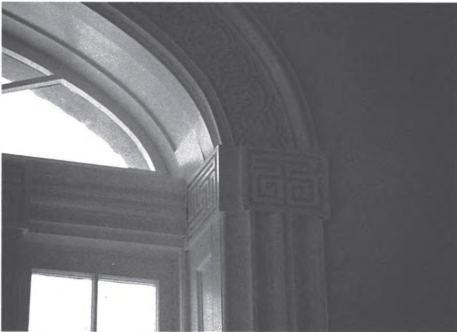
5-20. Greek fret composed of two spirals topped by an additional loop. Located at the springing of the arch over the west window, upper court. Compare the moldings to fig. 5-10.
