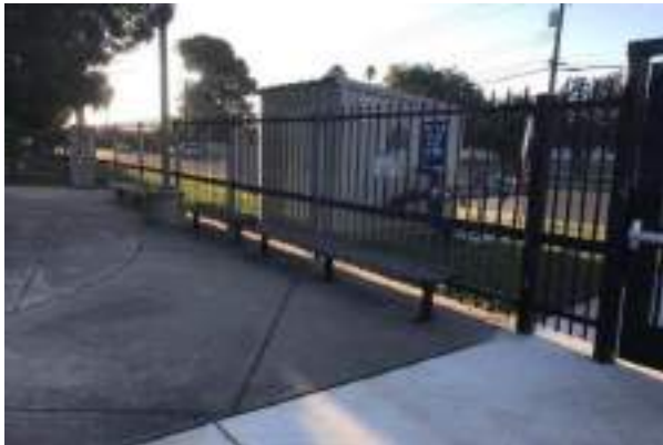
#3 DEFICIENCY FENCES & GATES, PAINTED SURFACE
