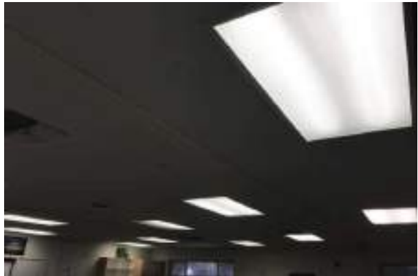
#64 LIGHTING SYSTEM, INTERIOR
