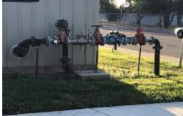
#32 BACKFLOW PREVENTER, DOMESTIC
