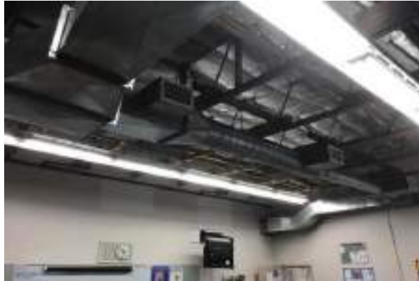
#55 HVAC SYSTEM DUCTWORK
