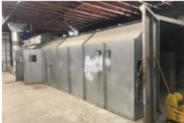
#75 PAINT SPRAY BOOTH
