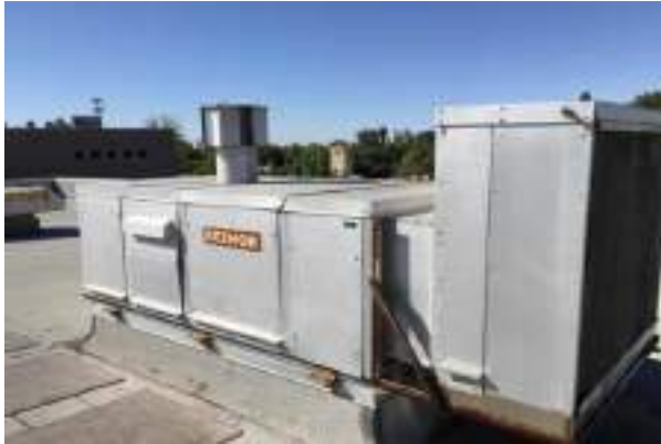
#49 MAKE-UP AIR UNIT
