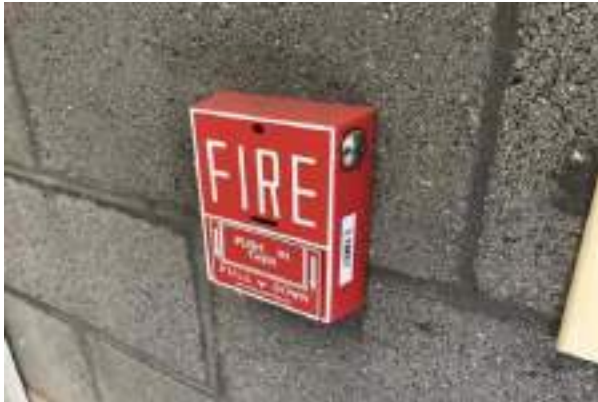
#71 FIRE ALARM SYSTEM
