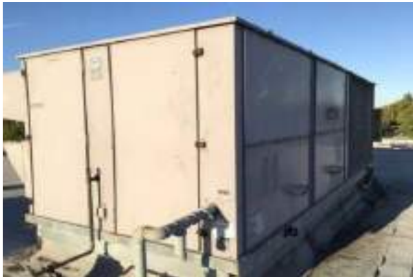
#51 PACKAGED UNIT (RTU)
