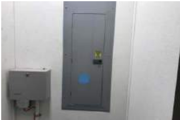
#65 MAIN DISTRIBUTION PANEL
