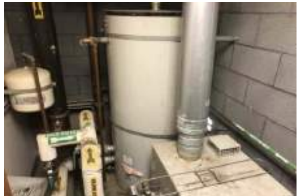
#42 WATER STORAGE TANK (FOR BOILER)
