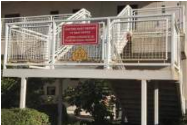
#5 DEFICIENCY G20 FENCES & GATES, PAINTED SURFACE
