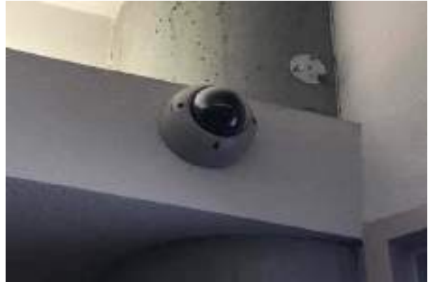
#74 SECURITY/SURVEILLANCE SYSTEM, CAMERAS AND CCTV
