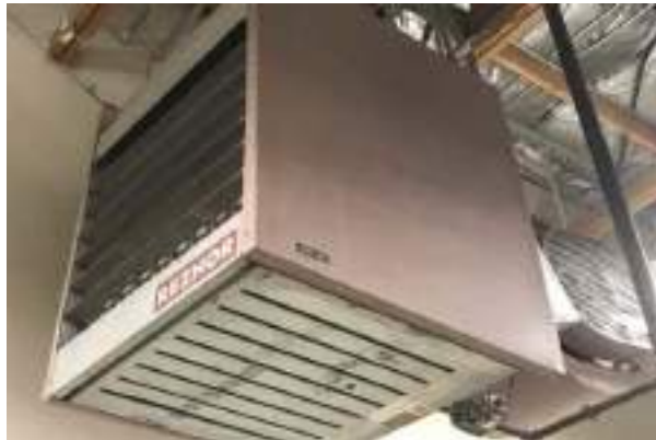
#57 UNIT HEATER, NATURAL GAS
