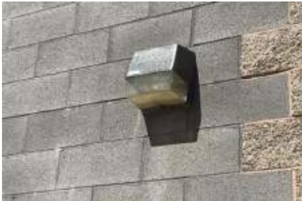
#63 LIGHT FIXTURE, EXTERIOR
