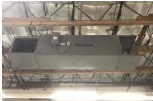
#58 DUST COLLECTION SYSTEM
