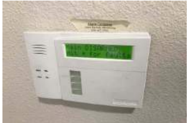
#72 INTRUSION DETECTION ALARM SYSTEM
