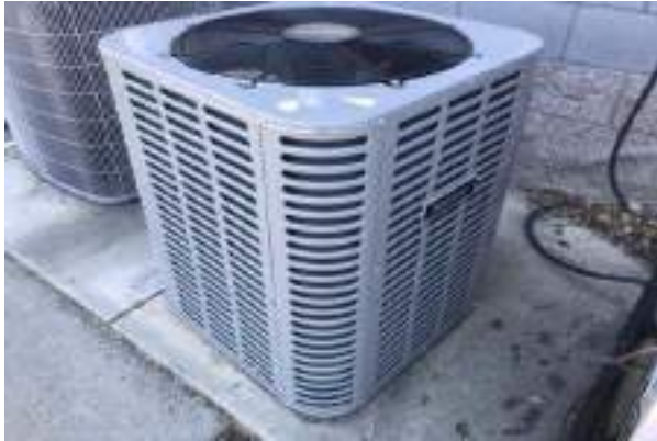
#43 CONDENSING UNIT/HEAT PUMP, SPLIT SYSTEM
