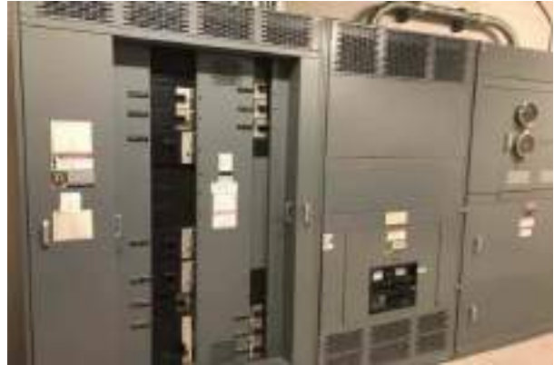
#68 SITE MAIN SWITCHBOARD
