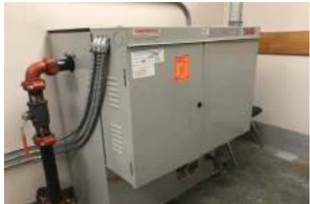
#30 ELEVATOR, HYDRAULIC MOTOR
