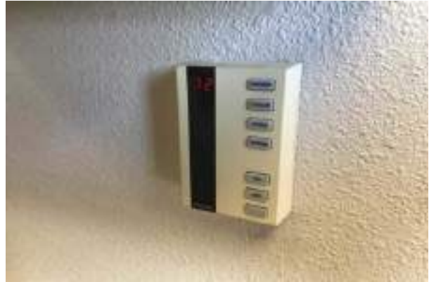
#2 DEFICIENCY EMS/BAS CONTROLS
