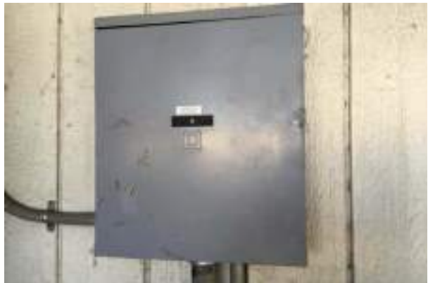
#66 MAIN DISTRIBUTION PANEL (PORTABLES)
