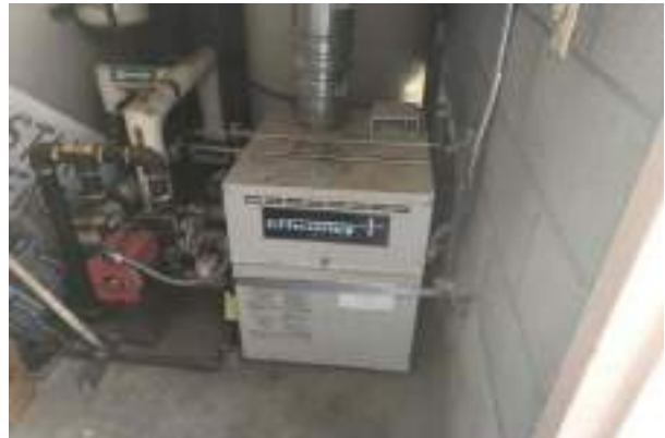
#40 DOMESTIC BOILER, GAS
