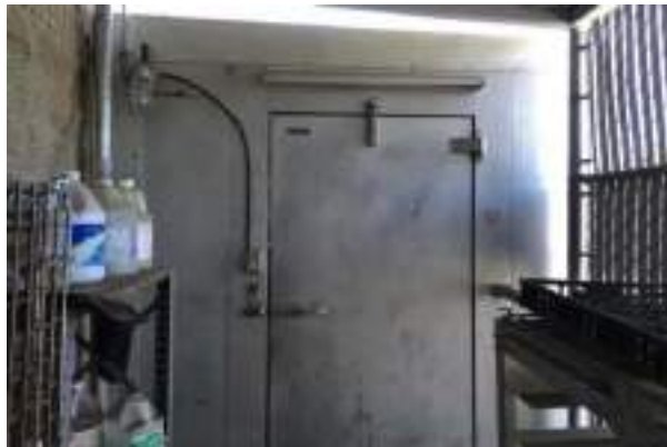
#77 COMMERCIAL KITCHEN, WALK-IN REFRIGERATOR/FREEZER
