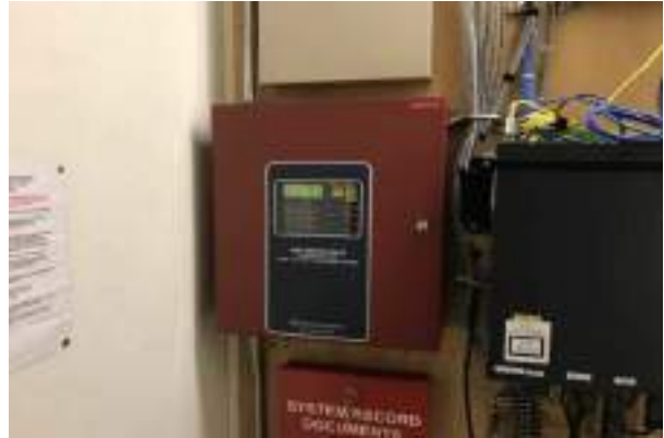
#70 FIRE ALARM CONTROL PANEL
