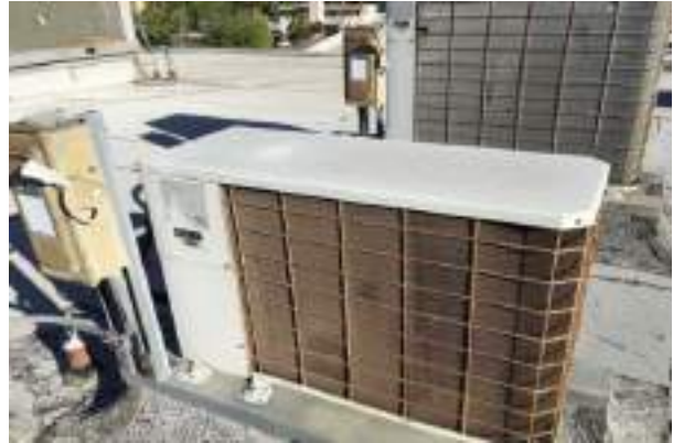
#44 CONDENSING UNIT/HEAT PUMP, SPLIT SYSTEM
