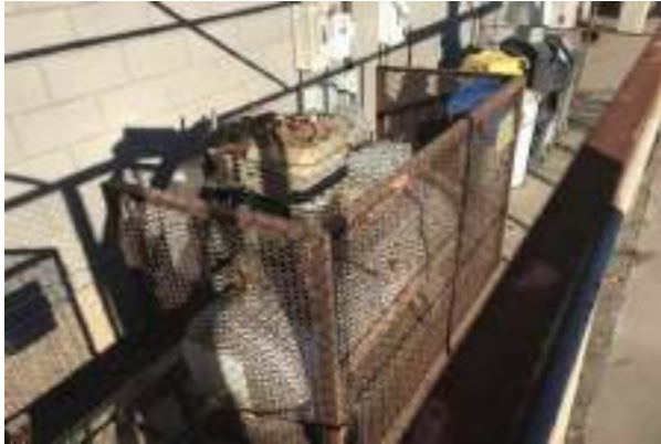
#1 DEFICIENCY AIR COMPRESSOR
