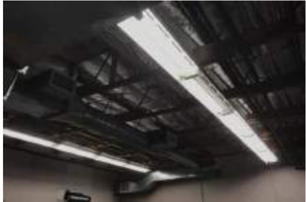
#62 INTERIOR LIGHTING SYSTEM
