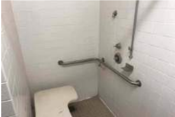
#7 DEFICIENCY SHOWER FIXTURES
