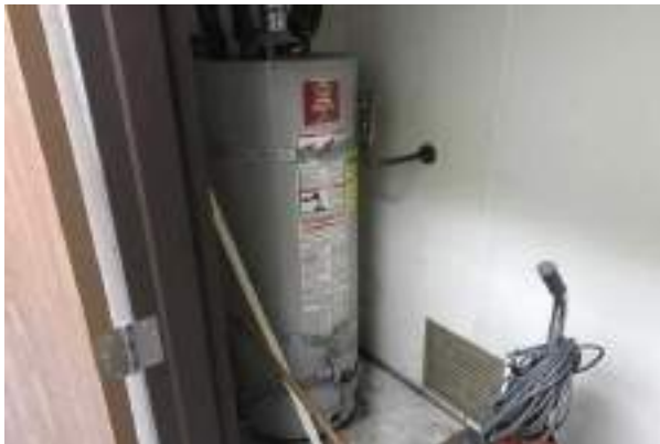
#41 WATER HEATER, GAS
