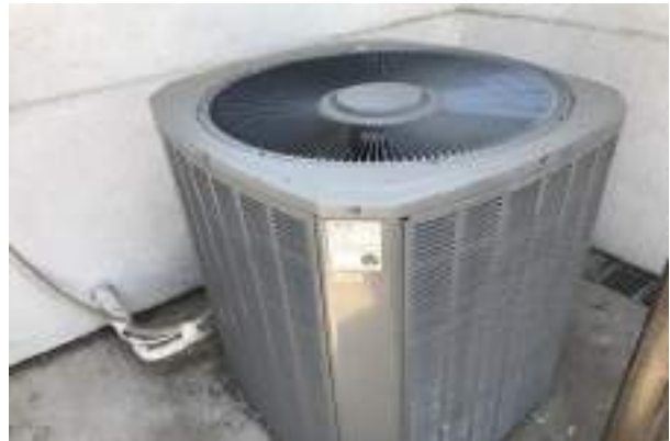
#28 CONDENSING UNIT/HEAT PUMP, SPLIT SYSTEM
