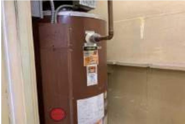
#19 GAS FIRED WATER HEATER
