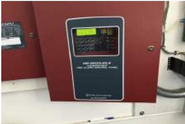
#21 FIRE ALARM CONTROL PANEL, BASIC/ZONED, REPLACE
