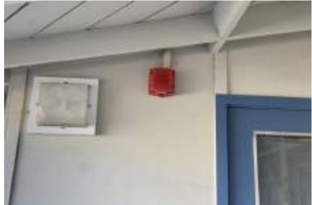
#20 FIRE ALARM SYSTEM
