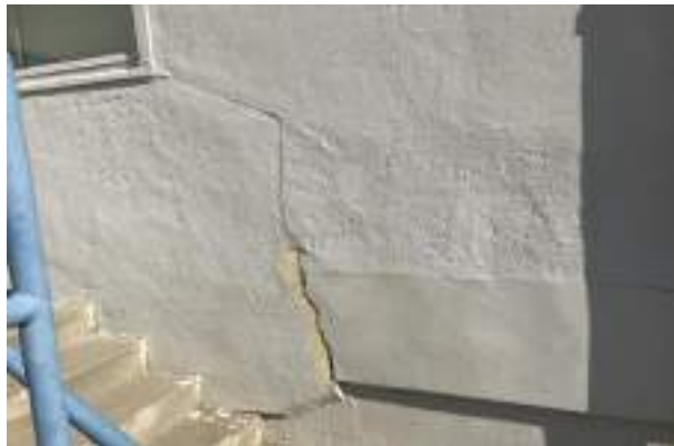
#36 ENGINEER, STRUCTURAL, SUPERSTRUCTURE, EVALUATE/REPORT. CRACKING NOTED AT 001 BUILDING (AU
