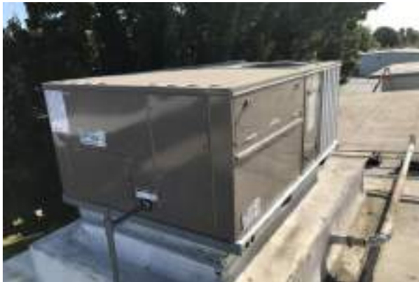
#27 PACKAGED UNIT (RTU)
