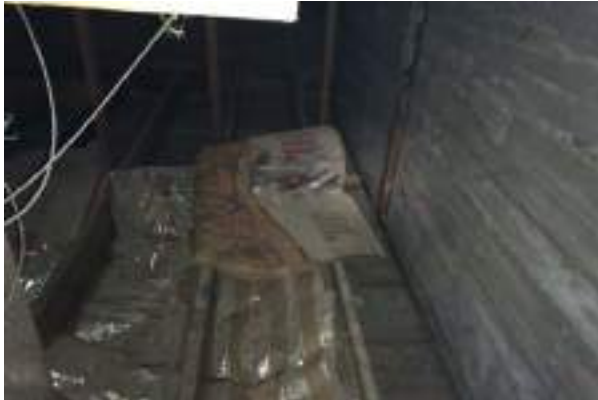
#45 FALLEN INSULATION FROM BUILDING A ATTIC
