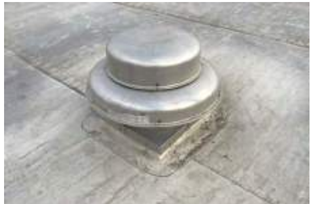
#60 BUILDING A, EXHAUST FAN
