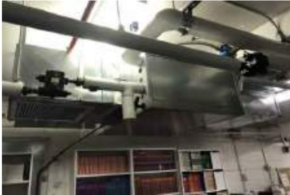
#73 FAN COIL TERMINAL UNIT, STEAM PIPING TO COIL
