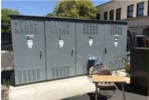
#61 BUILDING A, MAIN SWITCHGEAR, 277/480 V
