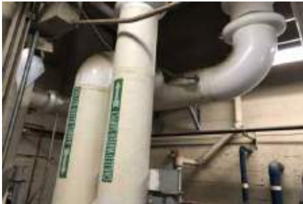
#75 CHILLED WATER PIPING
