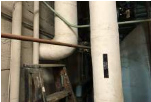
#63 DOMESTIC HOT WATER PIPING
