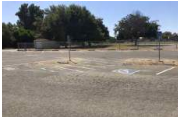
#78 PARKING LOT WITH ALLIGATOR CRACKING
