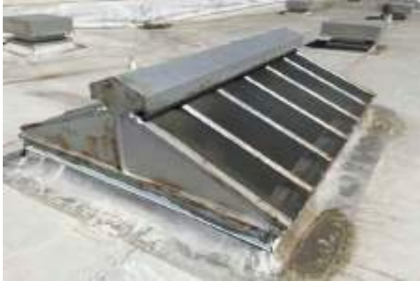
#19 BUILDING A SKYLIGHTS SHOWING SIGNS OF CORROSION AND AGE
