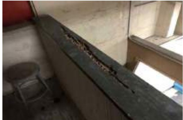
#48 DAMAGED INTERIOR WALL IN BUILDING C ATTIC
