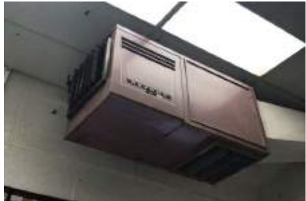
#58 BUILDING C FURNACE, GAS
