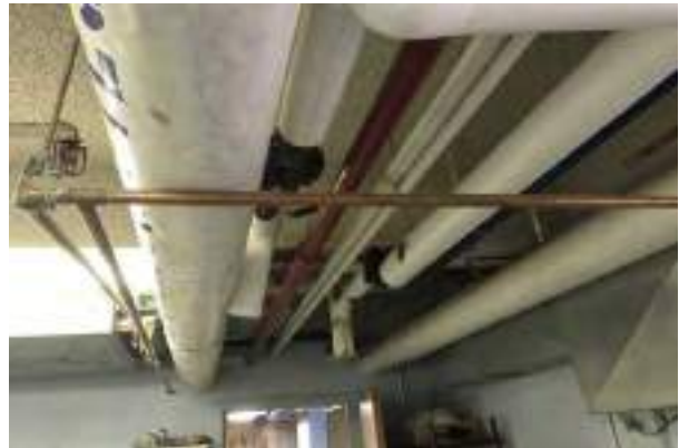
#64 HEATING HOT WATER DISTRIBUTION PIPING
