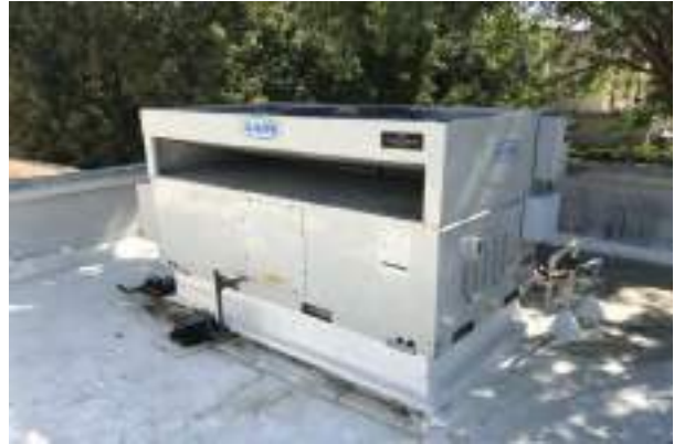
#56 BUILDING B PACKAGED UNIT (RTU)
