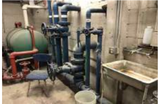
#74 BOILER ROOM DOMESTIC WATER PIPING
