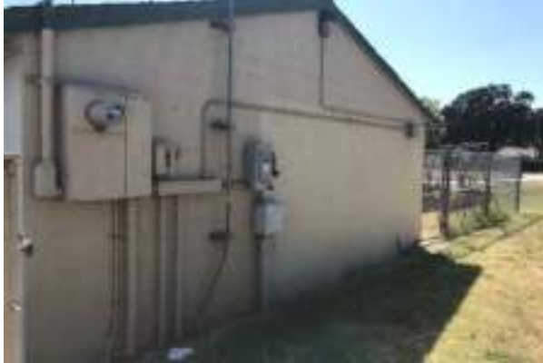
#67 ELECTRIC METER NEAR FOOTBALL FIELD
