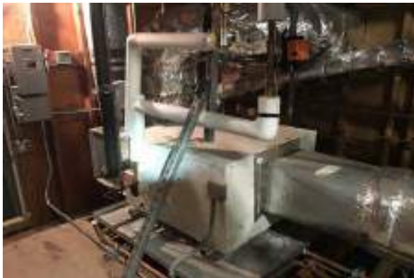
#59 BUILDING C AIR HANDLER (AHU)
