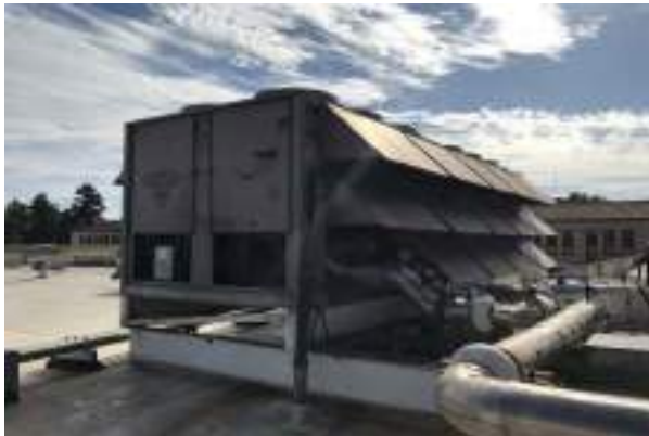
#57 AIR-COOLED CHILLER ON BUILDING A ROOF
