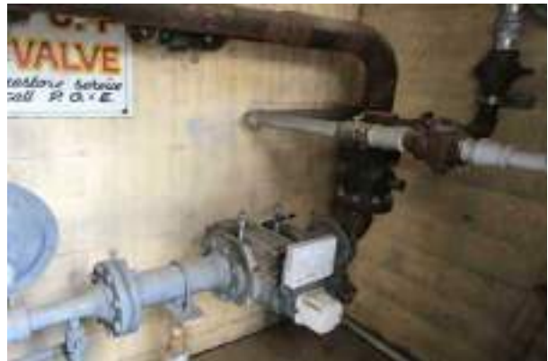
#66 NATURAL GAS METER
