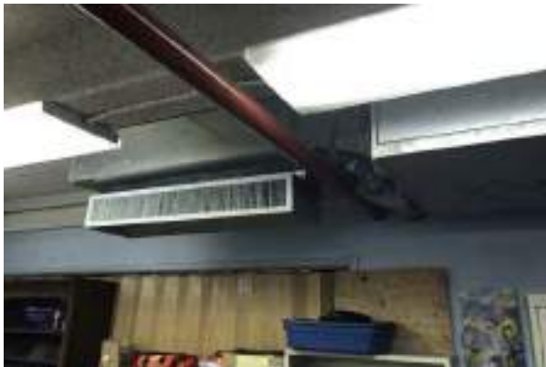
#65 BUILDING A, BASEMENT FAN-COIL UNIT
