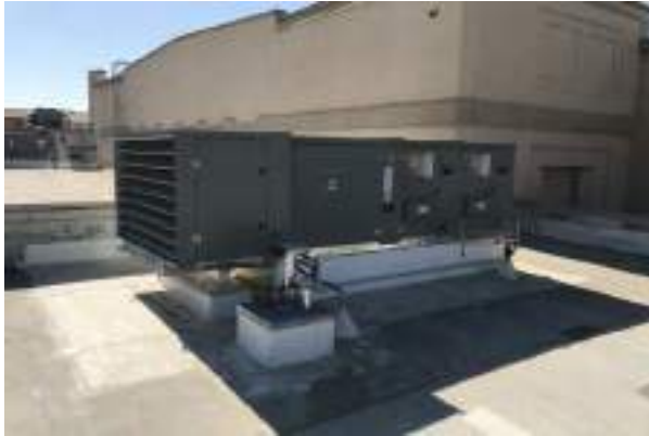
#55 BUILDING B FURNACE, GAS
