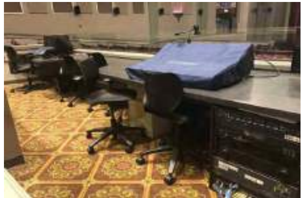
#30 THEATER CONTROL CENTER
