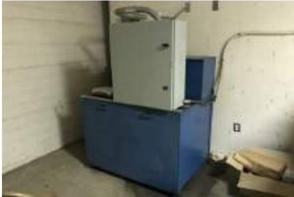
#49 HYDRAULIC ELEVATOR AND CONTROLLER
