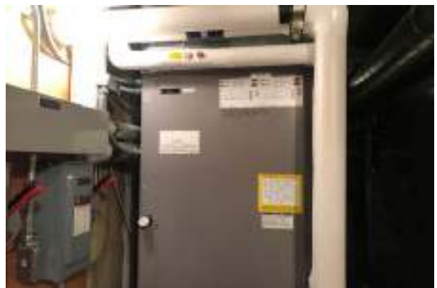
#24 AIR HANDLER (AHU), OFFICE
