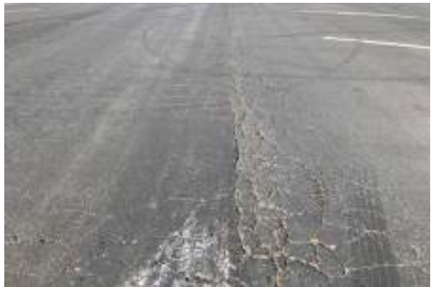
#52 DETERIORATED ASPHALT AT WEST PARKING LOT
