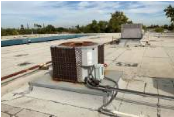
#25 ROOFTOP HVAC EQUIPMENT
