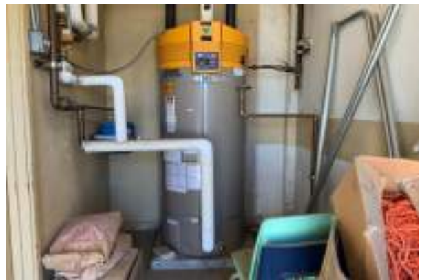
#22 GYM WATER HEATER
