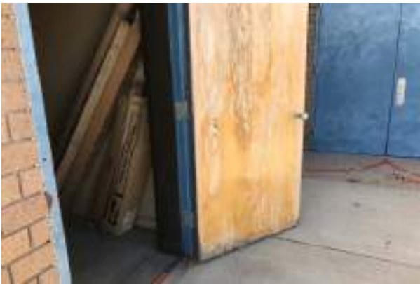
#45 DAMAGED DOOR AT GYM WATER HEATER ROOM
