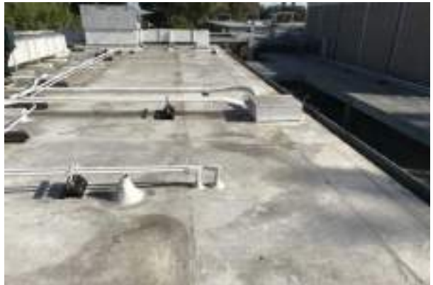
#22 TYPICAL MODIFIED BITUMEN ROOFING WITH REFLECTIVE COATING
