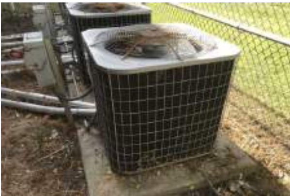
#33 CONDENSING UNITS-002 CLASSROOMS
