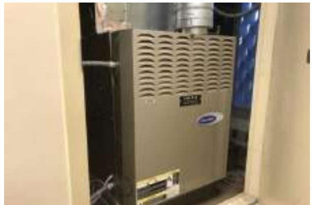
#34 INDOOR FURNACE-002 CLASSROOMS
