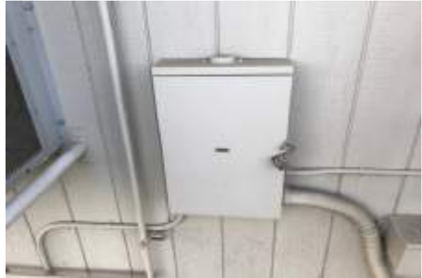
#38 PORTABLE MAIN DISTRIBUTION PANEL
