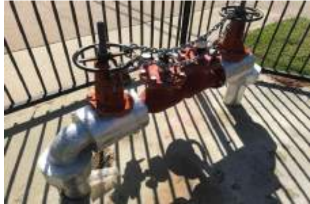
#26 BACKFLOW PREVENTER, DOMESTIC, 4"
