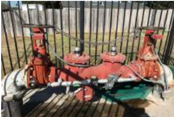
#27 BACKFLOW PREVENTER, FIRE PREVENTION, 8"
