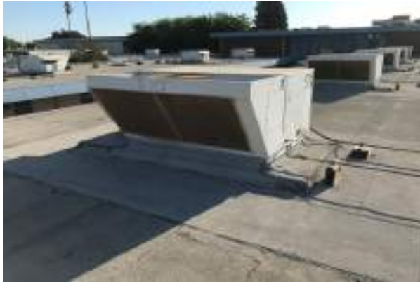
#31 PACKAGED UNIT (RTU)
