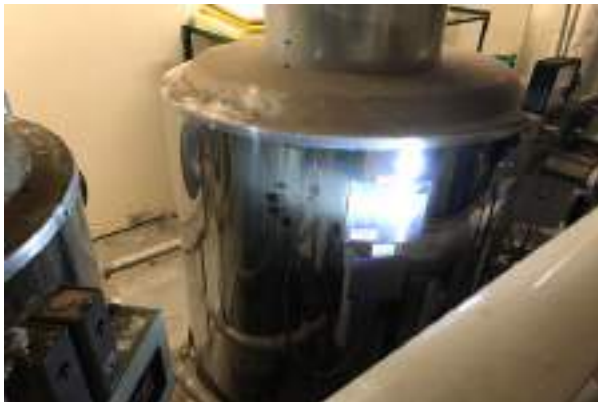
#29 DOMESTIC BOILER, GAS
