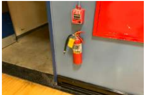
#36 FIRE ALARM SYSTEM
