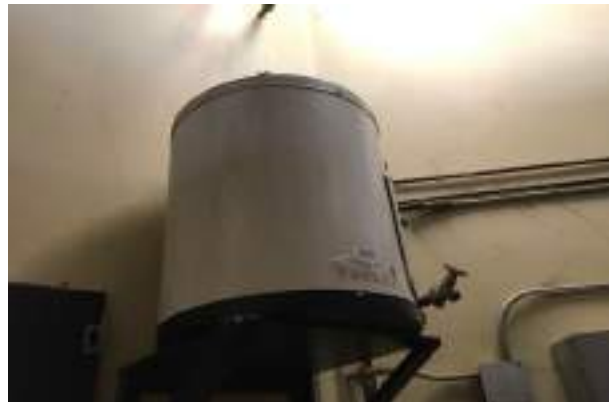
#30 WATER HEATER, ELECTRIC, RESIDENTIAL
