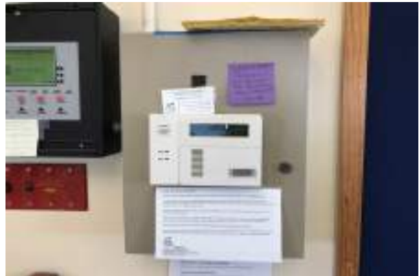
#40 SECURITY/SURVEILLANCE SYSTEM, CAMERAS AND CCTV
