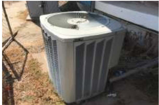
#34 CONDENSING UNIT, SPLIT SYSTEM
