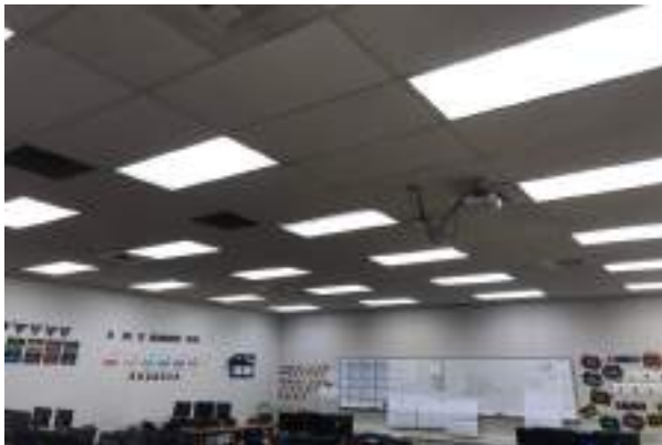
#41 INTERIOR LIGHTING SYSTEM
