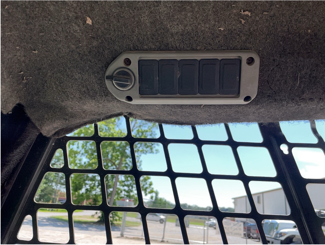
Switches and Controls / 05-15-2024
