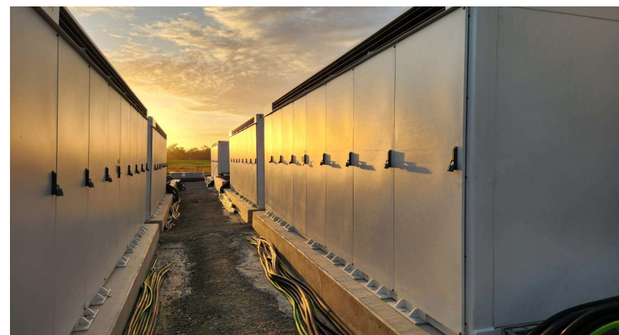
Figure 2: Tesla Megapacks at BBP Project
