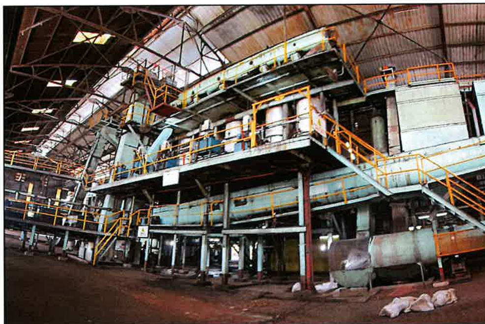
VIEW OF PRESS STATION
