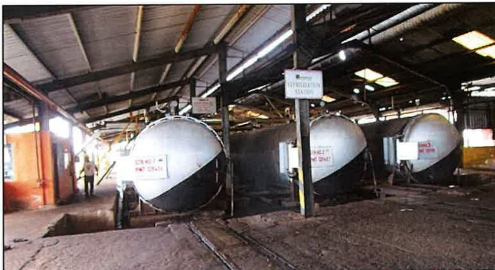
VIEW OF STERELISATION STATION
