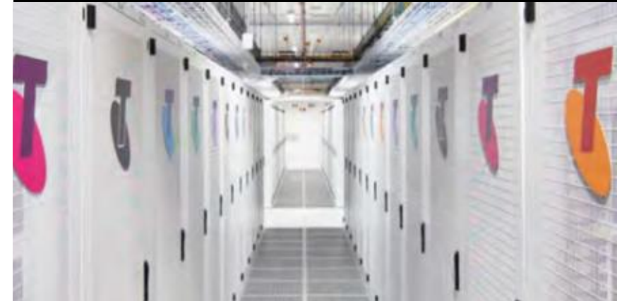
TELSTRA DATA CENTRE, CLAYTON VIC
