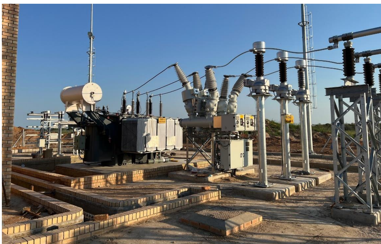
Lesedi Substation – Q1 2025
