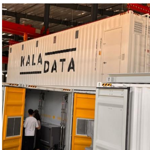
Data Centre Facility
