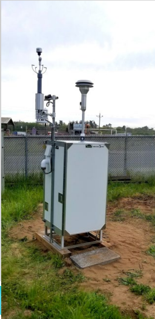
Weather Proof Enclosure at the OCSD
