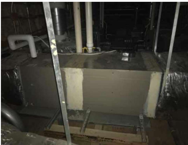
23 - SPLIT SYSTEM FAN COIL
