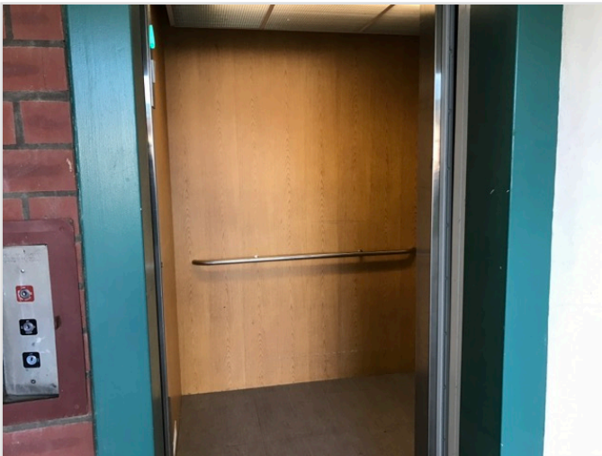
Lobby looking at cabs (with doors open)
