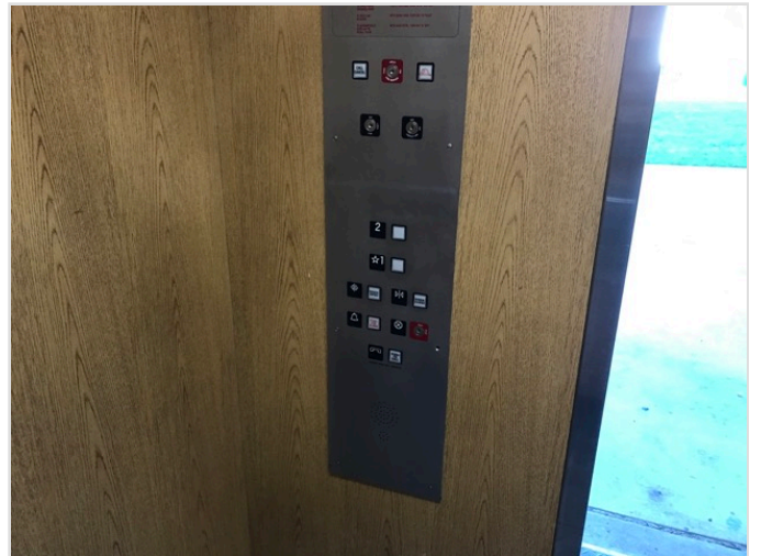
In-cab controls/emergency call panel
