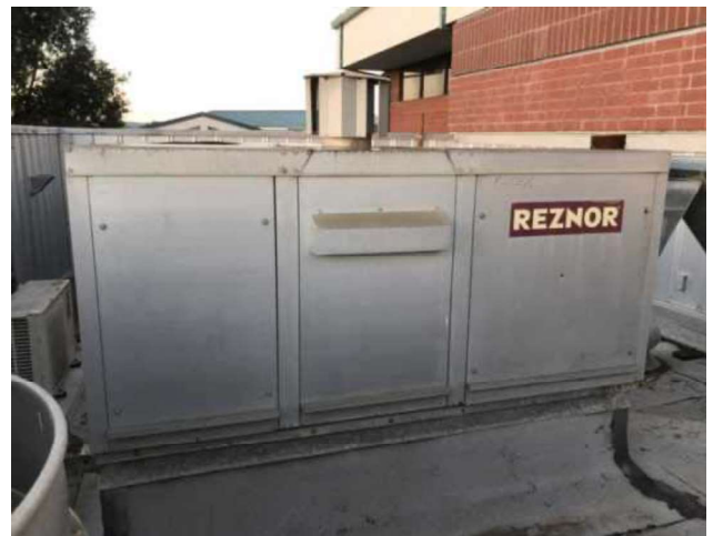
24 - MAKE UP AIR UNIT
