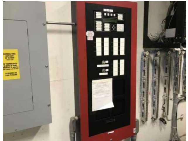
26 - FIRE ALARM PANEL
