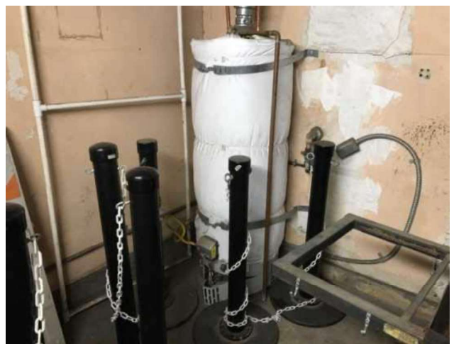
30 - WATER HEATER, BUILDING 050
