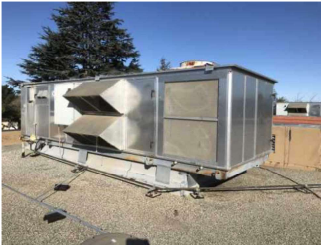
27 - AIR HANDLER, BUILDING 010
