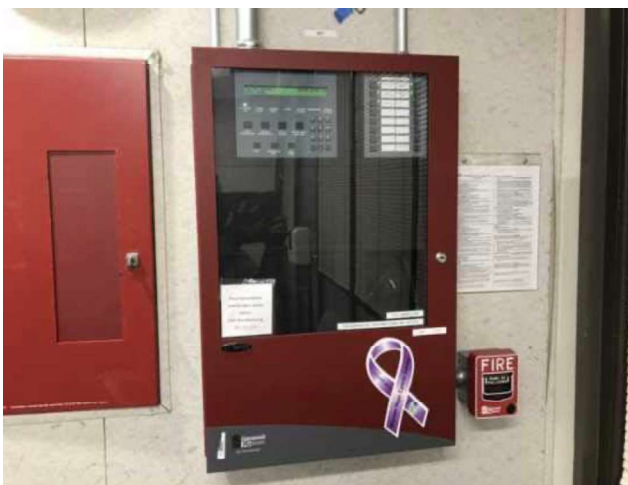
29 - FIRE ALARM PANEL, BUILDING 010
