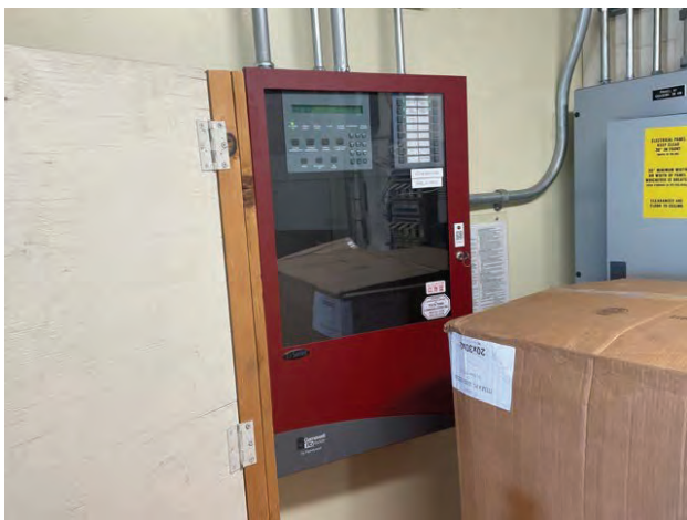
17 – FIRE ALARM PANEL
