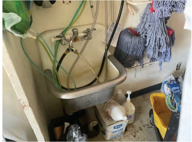
14 – SINK AND PLUMBING
