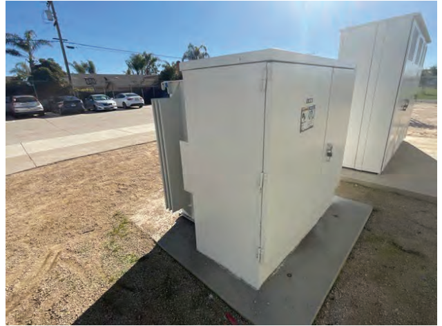
20 – TRANSFORMER AND SWITCHBOARD
