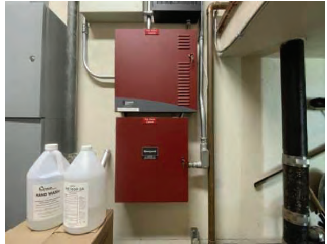
26 - FIRE ALARM PANEL
