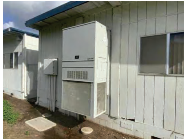
22 - ANCILLARY BUILDING HVAC UNIT
