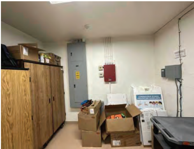
21 - MAIN ELETRICAL EQUIPMENT
