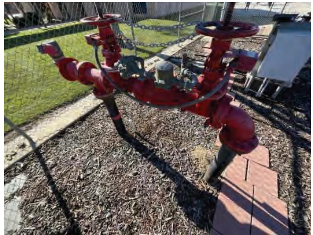
22 - FIRE SUPPRESSION BACKFLOW PREVENTER
