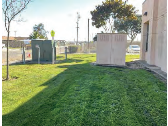
20 - MAIN ELETRICAL EQUIPMENT
