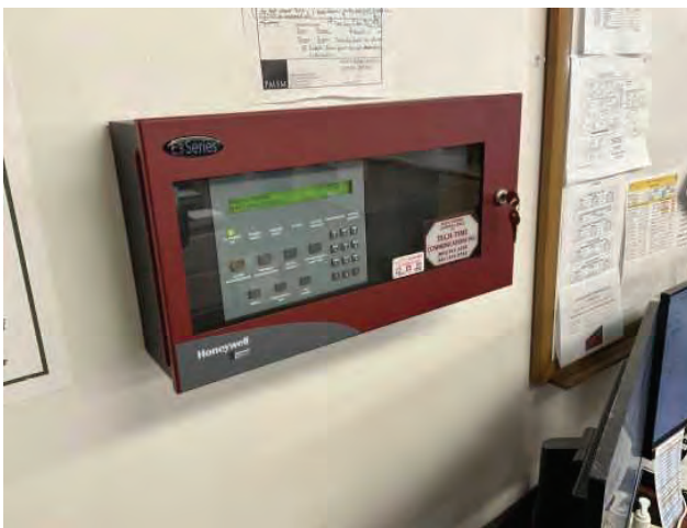
23 - FIRE ALARM PANEL
