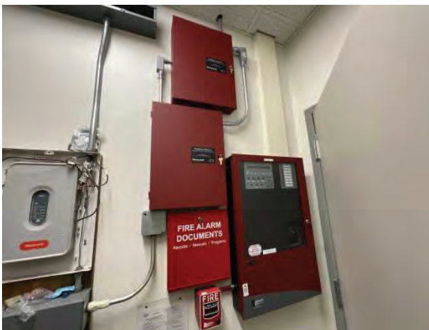
23 - FIRE ALARM PANEL
