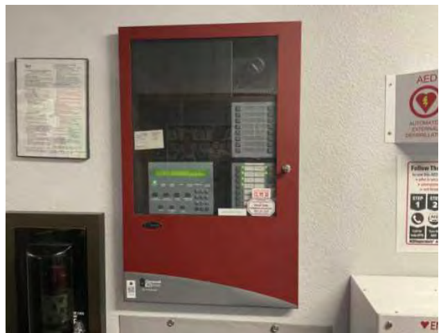
30 - FIRE ALARM PANEL
