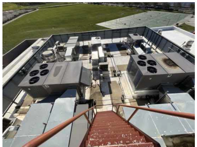
18 - HEATING MAIN COMPONENTS / AHU
