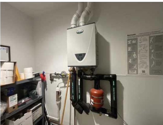
17 - DOMESTIC WATER HEATER
