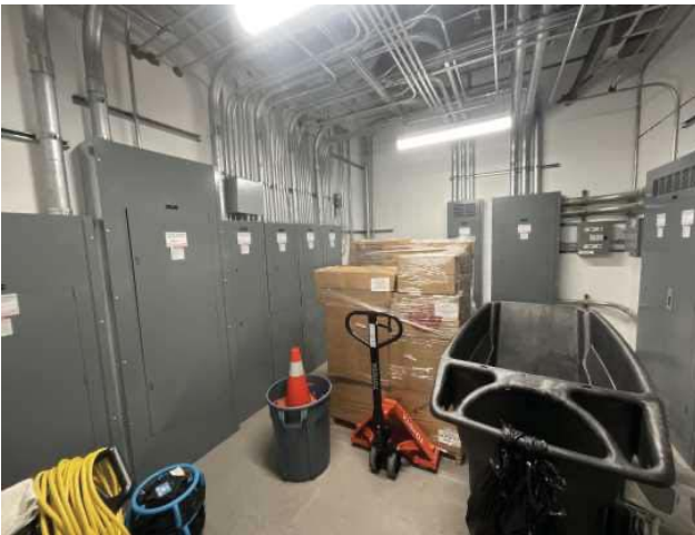
21 - MAIN ELETRICAL EQUIPMENT
