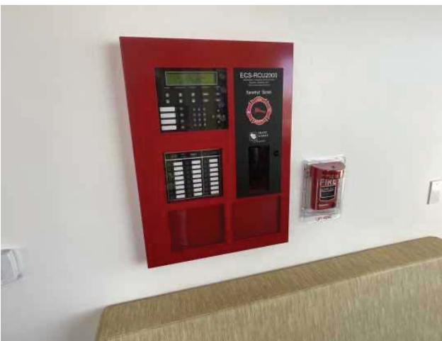
23 - FIRE ALARM PANEL
