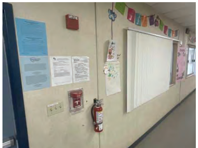
30 - FIRE ALARM SYSTEM
