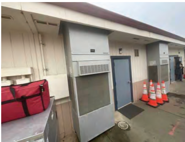
23 - WALL-MOUNTED HEAT PUMP
