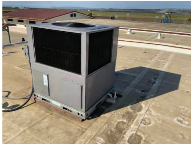
22 - PACKAGED ROOFTOP UNIT
