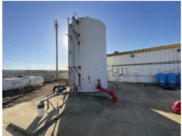
20 - WATER STORAGE TANK
