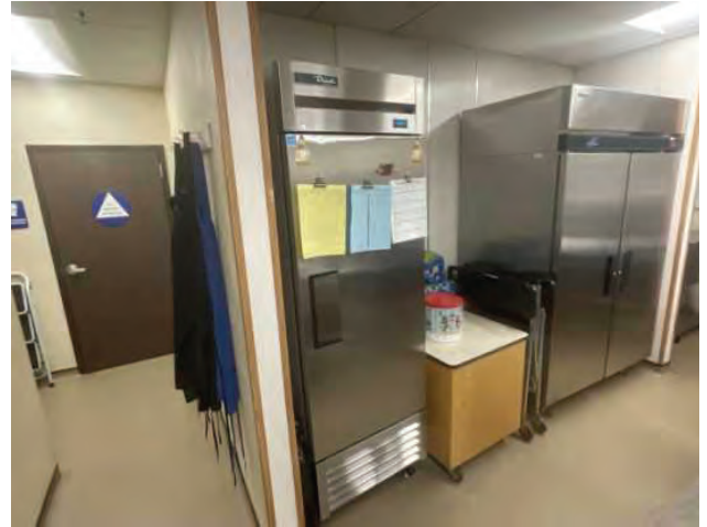
32 - REACH-IN REFRIGERATION UNITS
