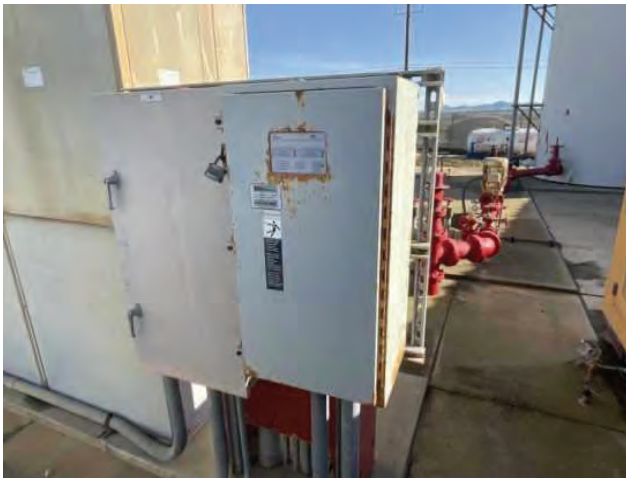
27 - AUTOMATIC TRANSFER SWITCH
