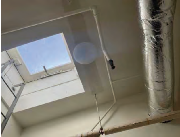
25 - FIRE SUPPRESSION SYSTEM
