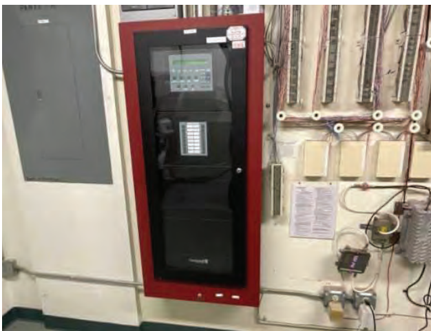
29 - FIRE ALARM PANEL
