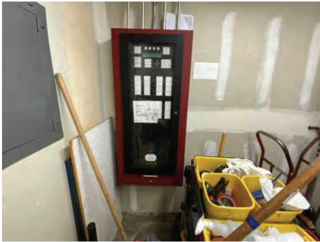
37 – FIRE ALARM PANEL
