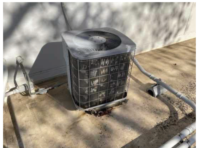
18 - SPLIT SYSTEM HEAT PUMP
