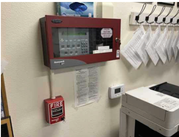
23 - FIRE ALARM PANEL
