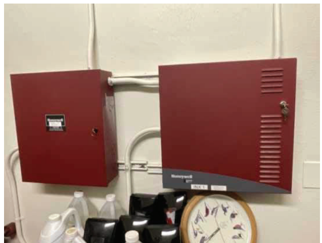
24 - FIRE ALARM BOOSTER PANEL
