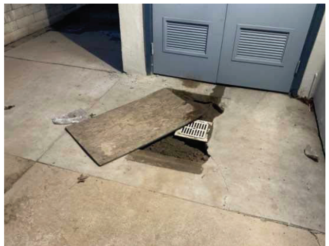
36 - CONCRETE FAILURE, TRIP HAZARD
